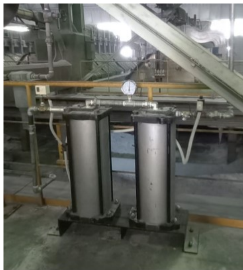
Figure 10. Air tank in Auto Retract installation.
